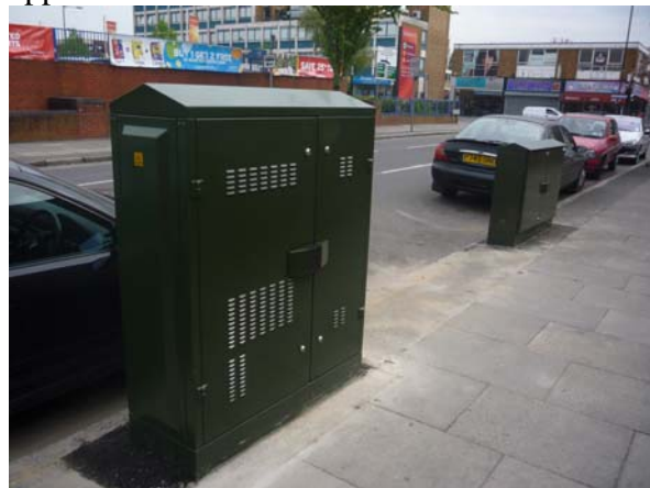
Large telecoms boxes add to street clutter
